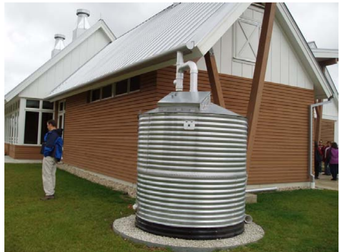
Figure 3.3b: Above Grade Cistern
